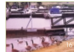
Not high enough, posts spaced too far apart
